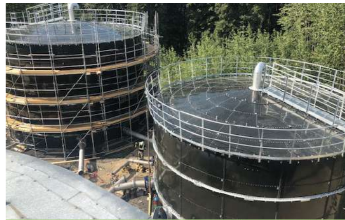
Potable Water Storage Tanks in Canada
