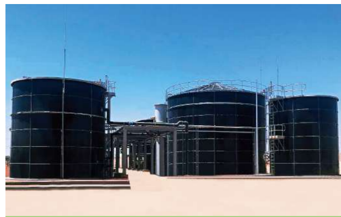
Coca Cola Plant Wastewater Treatment Plant
