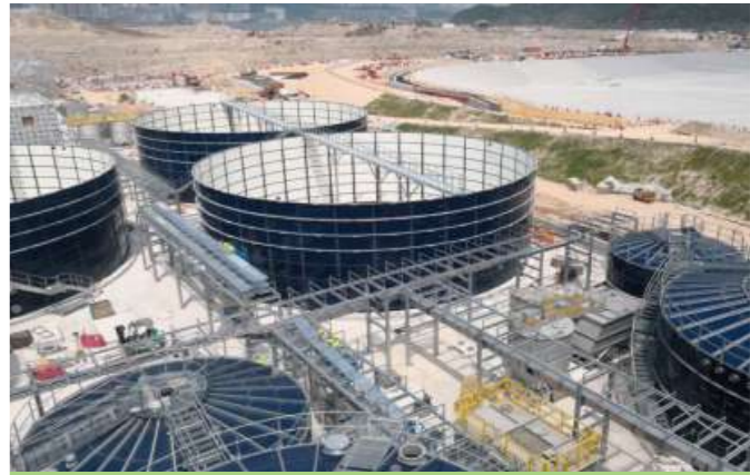
Veolia Landfill Leachate Treatment Project
