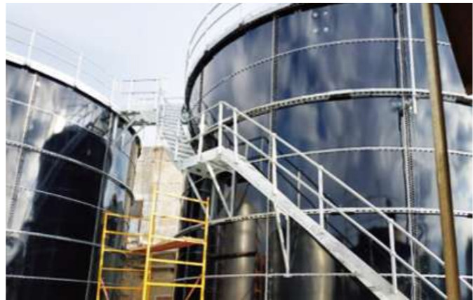
KuibyshevAzot Chemical Plant Wastewater Treatment
